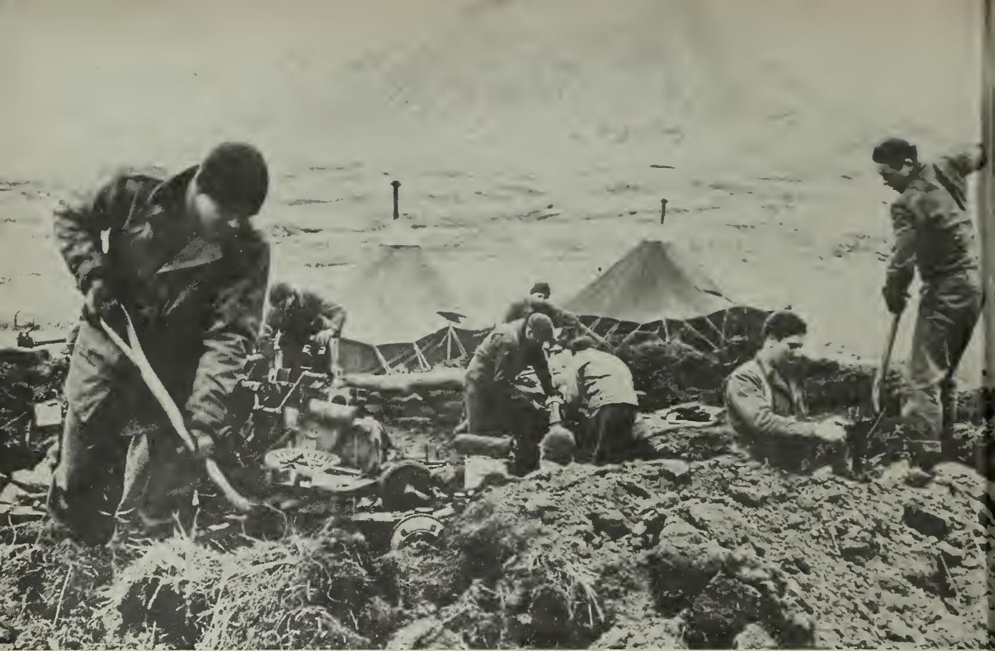
FIGHTING SEABEES built Pacific bases from Alaska to South Pacific. Here, CBs dig gun position on Attu Island.
